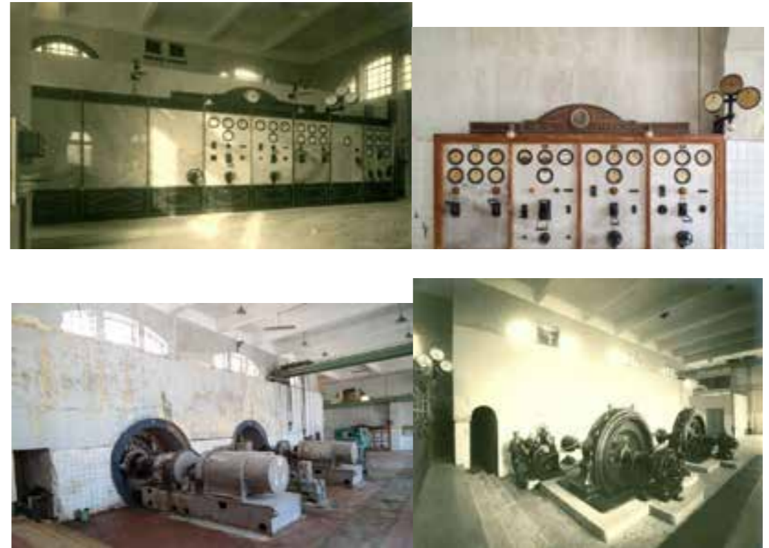
Figures 14-17 the old and new turbine motors at El Faiyum Power Station ©ShreenMohmed, January 9, 2020. & explore Fayoum, accessed May 31, 2020 https://fayoumgypt.com/explore-fayoum-with-fayoumer/
