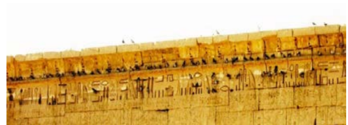
In holes, carved inscription, gaps, or crevasses, wherever they alight, their waste destroys and defaces the fabric and decoration of the ancient structures
